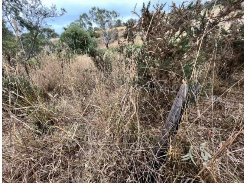
Photo 3. Inappropriate barb wire fence inside conservation area
