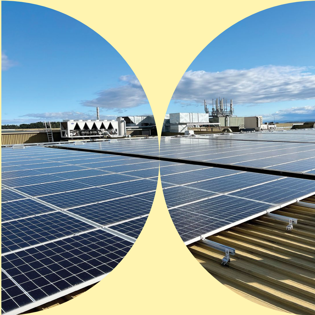
Chirnside Park, VIC, solar PV array
